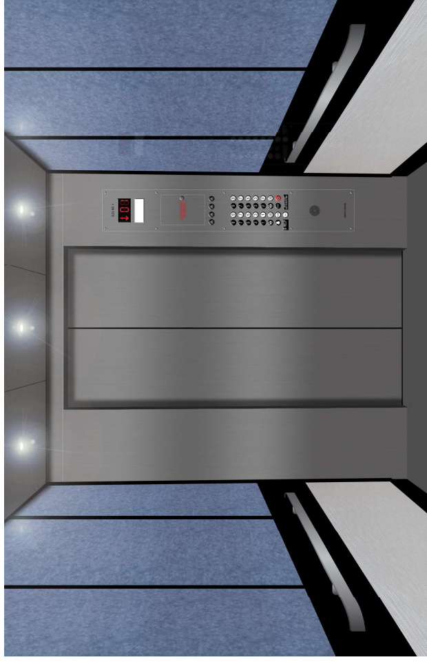
Pictured: Belair with top panels Wilsonart® D502-18: Ocean, bottom panels Chemetal® 231 Metawave, LED downlights in stainless steel drop ceiling, 2" stainless steel flat hand rails with returns.
